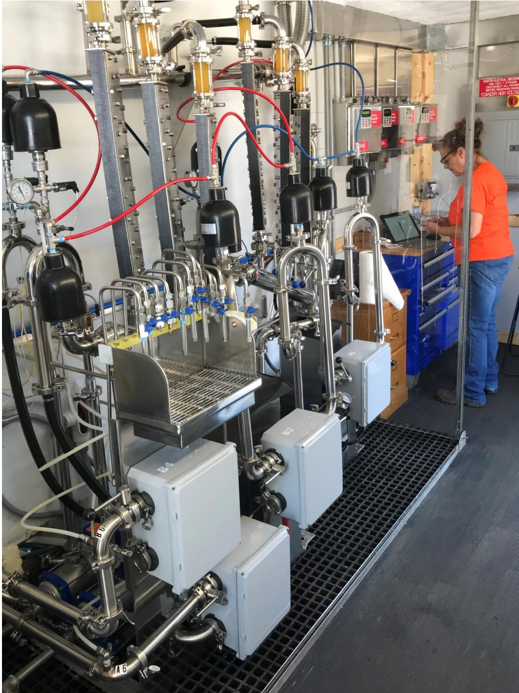
Operating AMEOX® Dual Unit destroying PFAS in GAC and removing iron at low power (<50amps), low pressure (<100psi) and ambient temperature (100oF). (Waste Recovery Systems, Inc., Wyoming, MI – June 2022)
